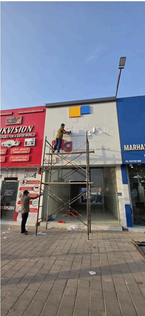
On site during installation
